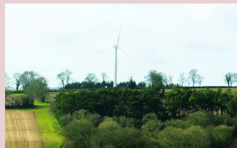
Electricity is fed to the community from the estate's 500kW wind turbine that sits high on a hill.
